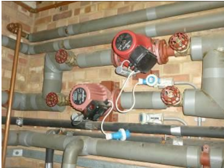
Photograph 6 – Care Home plant room heating circulating pumps and distribution pipework.
