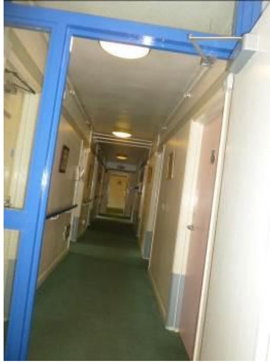
Photograph 1 – Care home example of corridor 2D compact lighting.
