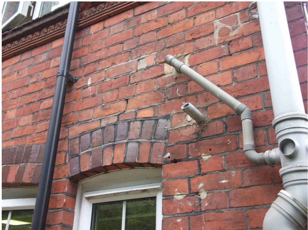
Photograph 08 (SVP pipe work)
