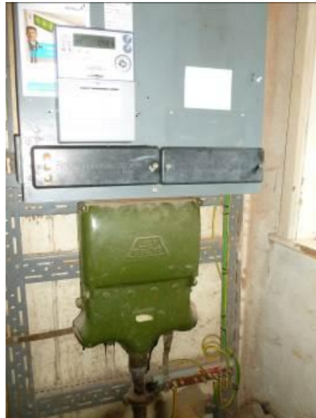
Photograph 4 – Care home main electrical incoming supply for both buildings.
