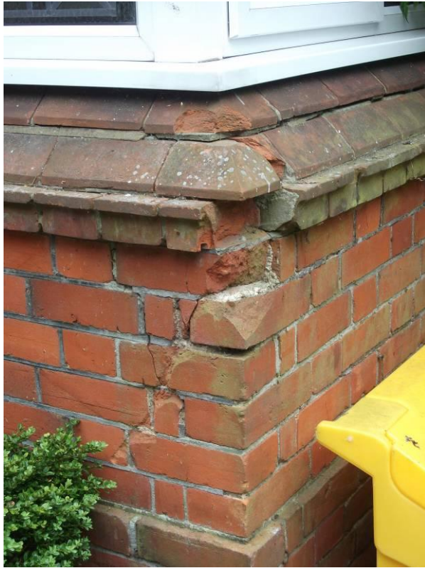
Photograph 05 (Entrance porch brickwork damage)
