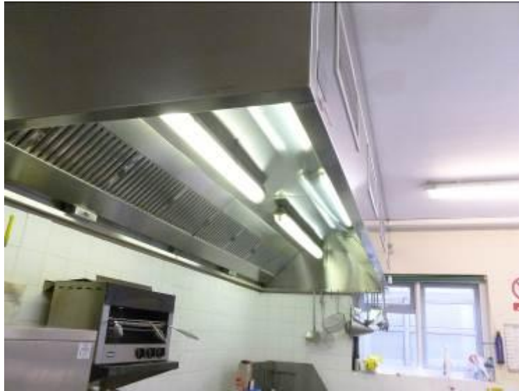
Photograph 5 – Care home new kitchen ventilation system.
