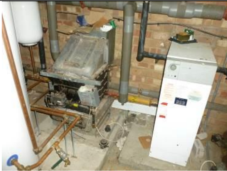
Photograph 7 – Care Home Potterton boilers life expired and de-commissioned.
