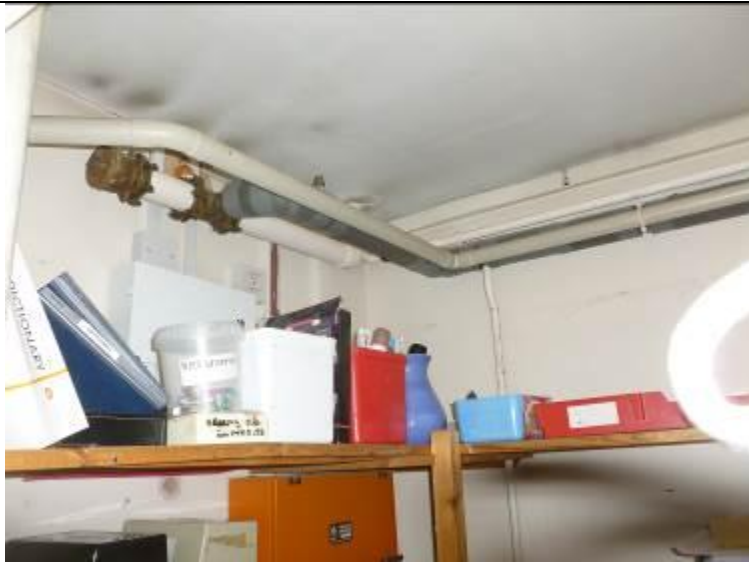
Photograph 11 – Example of distribution pipework.
