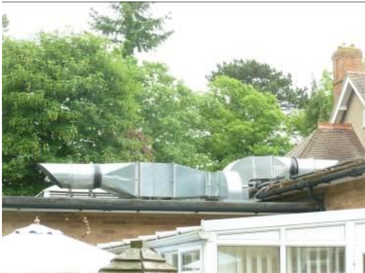
Photograph 14 – Roof mounted kitchen ventilation plant.
