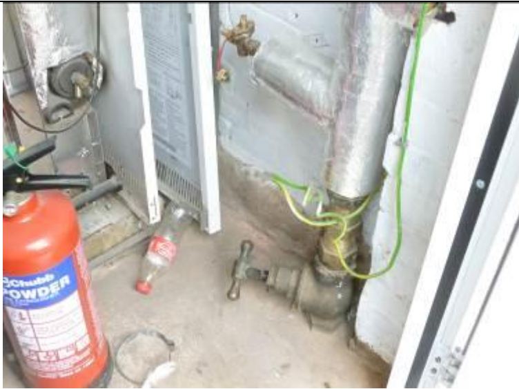
Photograph 13 – Main incoming water supply, note possible dead leg and earth bonding issue.
