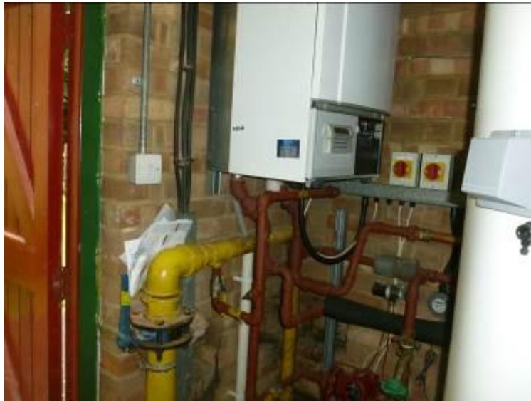
Photograph 9 – Care home more recently installed Broag gas fired boiler
