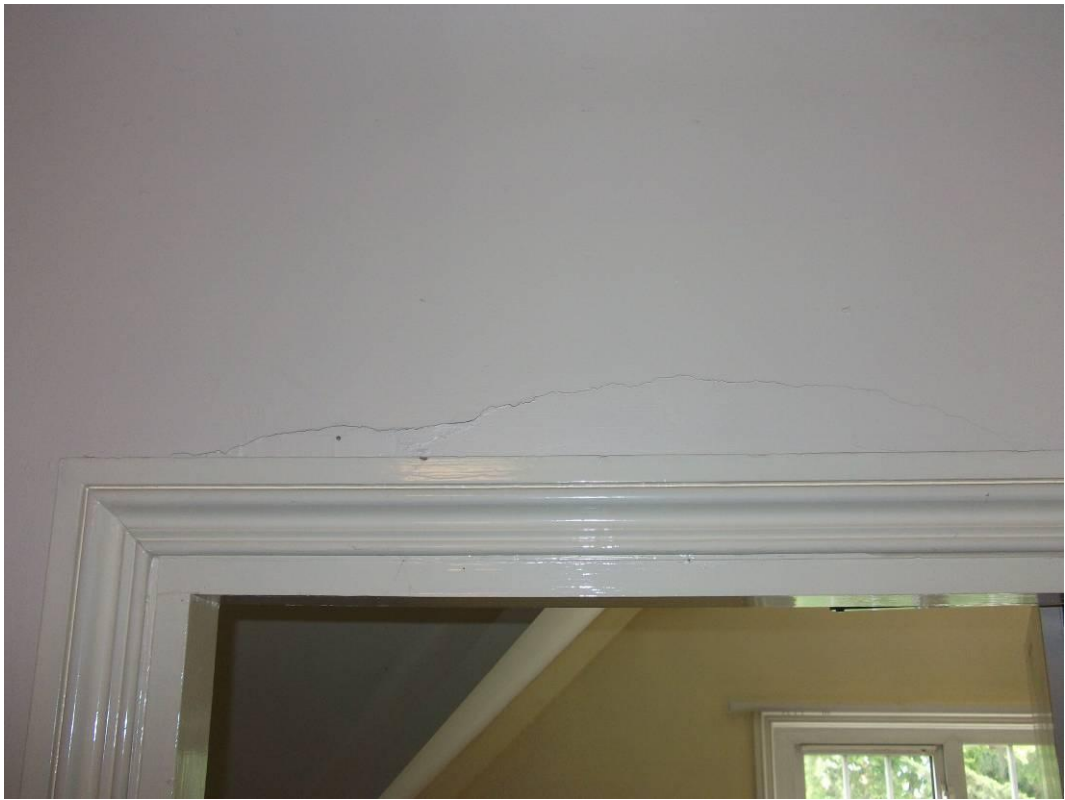
Photograph 11 (Crack above door second floor)
