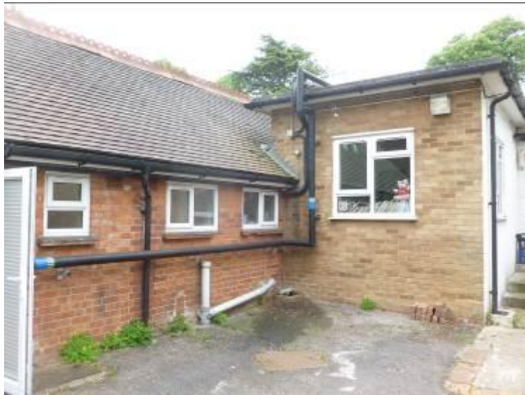
Photograph 12 – External distribution pipework extending to tank room.
